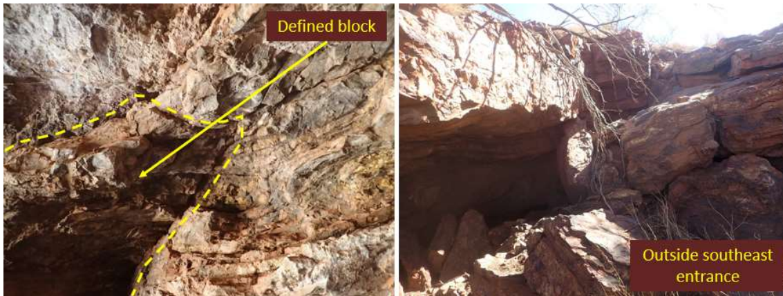
Figure 13 – Left hand photo shows an example of a well-defined block. Right hand photo shows the condition of the southeast brow and blocks outside the entrance
