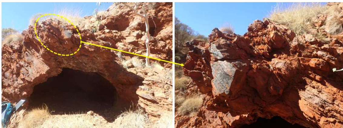
Figure 14 – View of the cave entrance and complete brow on the left. Right hand photo shows some of the cracking and dilation in the front part of the brow
